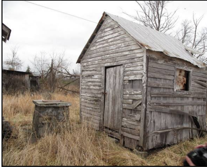
Figure 4. 2 Meathouse at CN-24. Note the horizontal weatherboards over the vertical board boxing. A raised cistern is located at left in photo.
